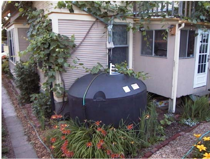
Figure 4-5 Residential Aboveground Cistern in Portland, Oregon ( www.rwh.in )
