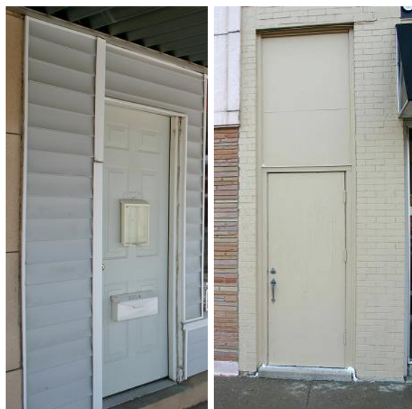
Inappropriate replacement doors and windows detract from the character of historic architecture and diminish the street-level appeal that distinguishes downtown Newton.
