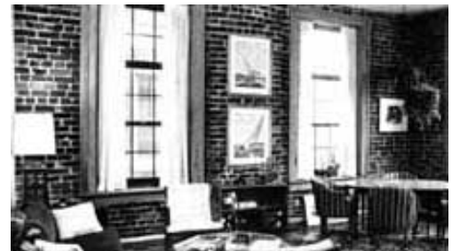
Plaster has been removed from perimeter walls, leaving brick exposed. The plaster should have been retained and repaired, as necessary. Photo: NPS files.
