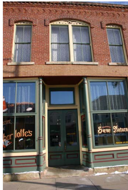
Cast-iron posts and wooden materials such as the ones that enframe these display windows are a common feature of historic storefronts. Existing storefront elements in downtown Newton should be retained.
