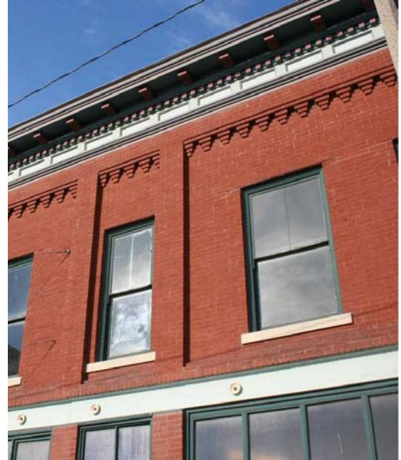
Features such as roof cornices with modillions and dentil moulding, as well as facade elements such as brick corbelling, should be retained. These should not be covered or removed.
