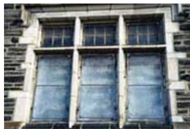
BEFORE: Example of deteriorated window conditions.
