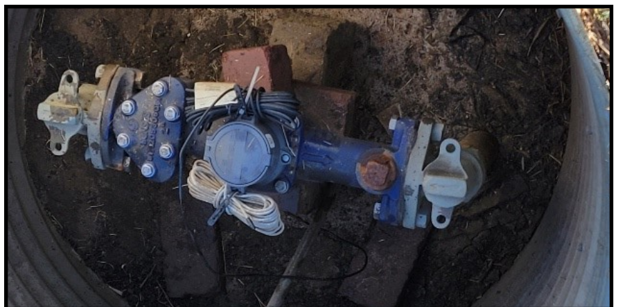
Meter Pit 2-inch
