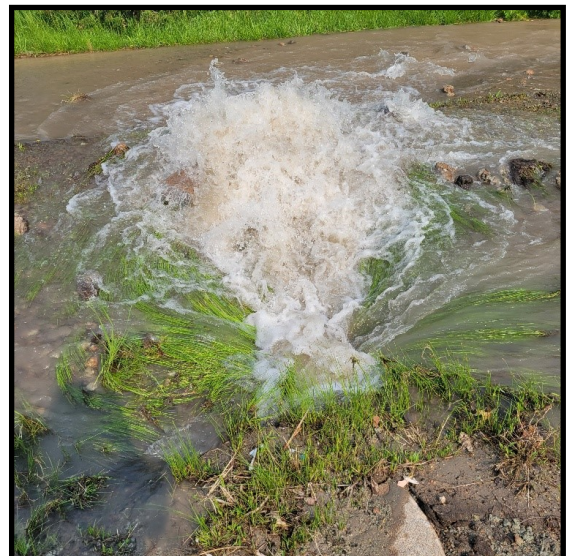
Main break at South Kansas and 24th Street
