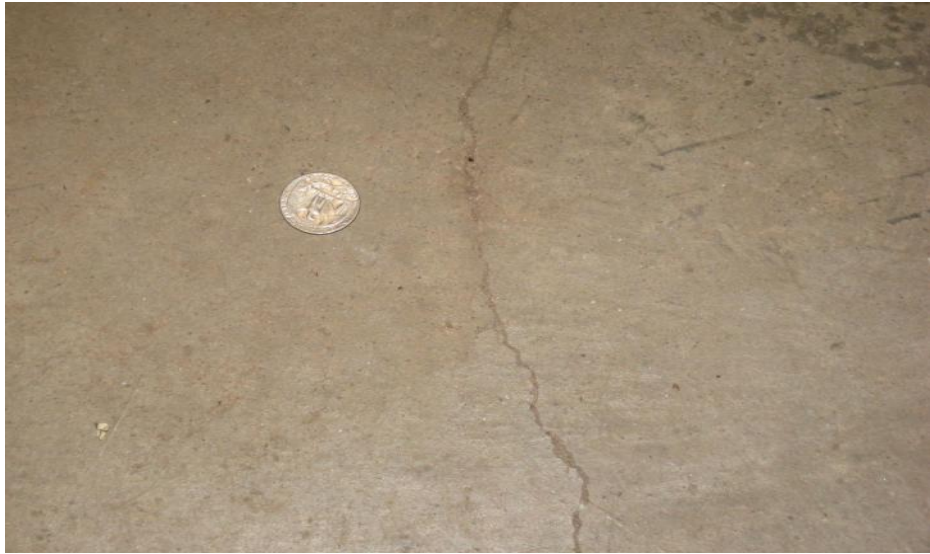
PHOTO 1 SLAB ON GRADE CRACKING AT BASEMENT
