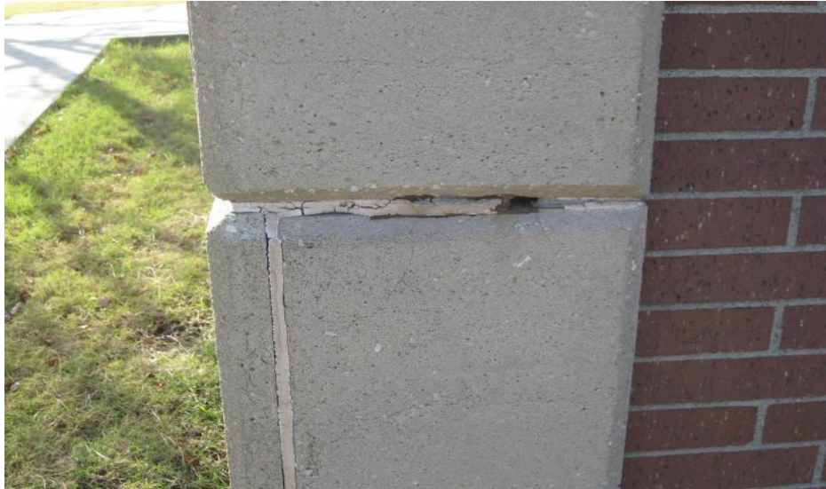
PHOTO 31 CRACKED PRECAST VENEER AT ADDITION AND SEALANT FAILURE
