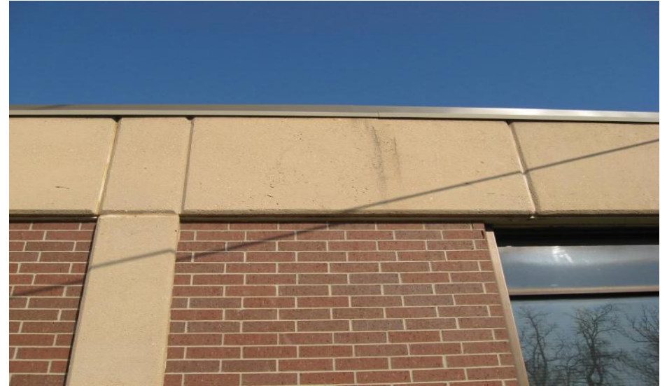
PHOTO 32 STAINING OF PRECAST VENEER AT CONCRETE CRACK LOCATIONS
