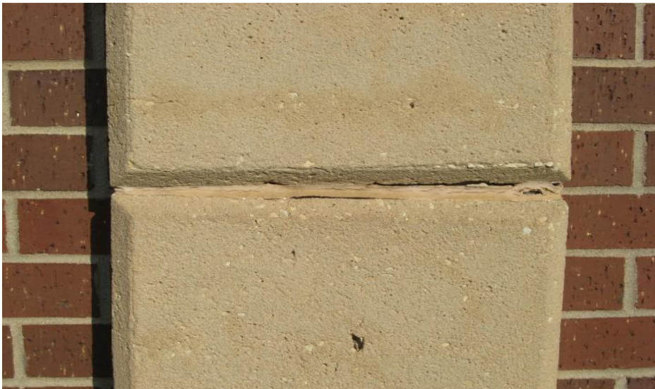
PHOTO 35 SEALANT FAILURE AT PRECAST VENEER
