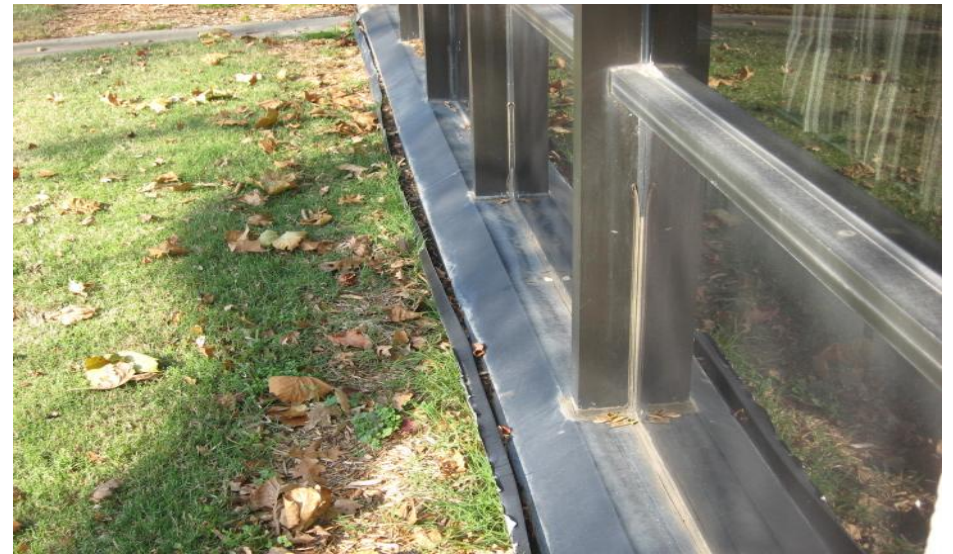
PHOTO 16 MODIFIED WINDOW FLASHING WITH GUTTER TO SPLASH BLOCK
