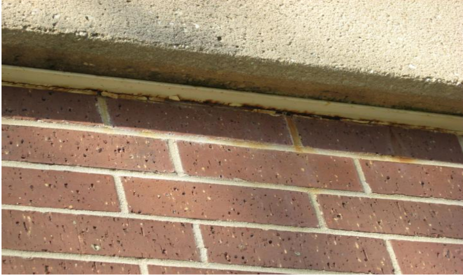
PHOTO 37 RUSTING VENEER LINTEL (NO DRIP ON PRECAST VENEER)
