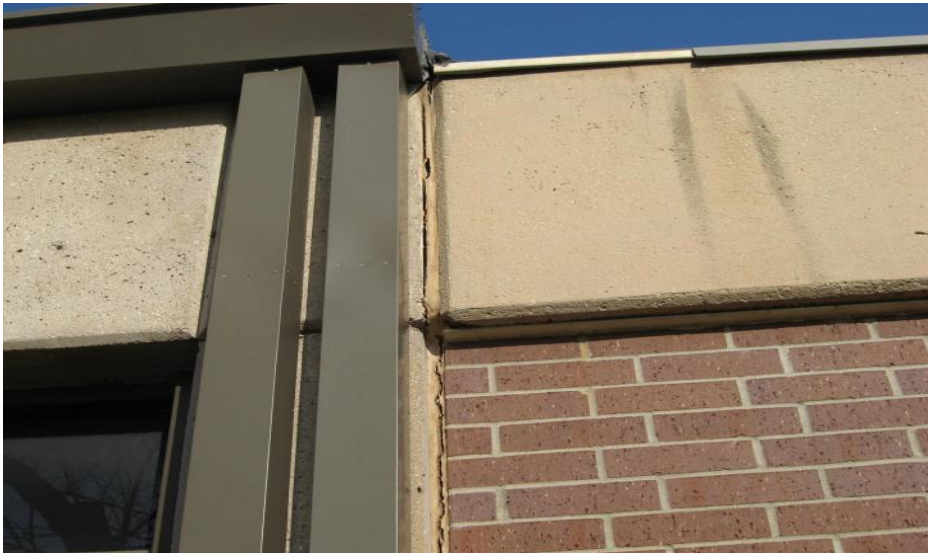
PHOTO 39 SEALANT FAILURE AT JOINT BETWEEN ORIGINAL BUILDING AND ADDITION
