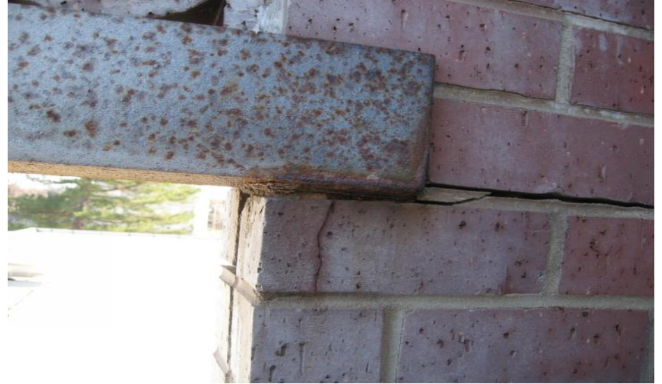
PHOTO 26 RUSTED LINTEL BEARING AND JOINT EXPANSION
