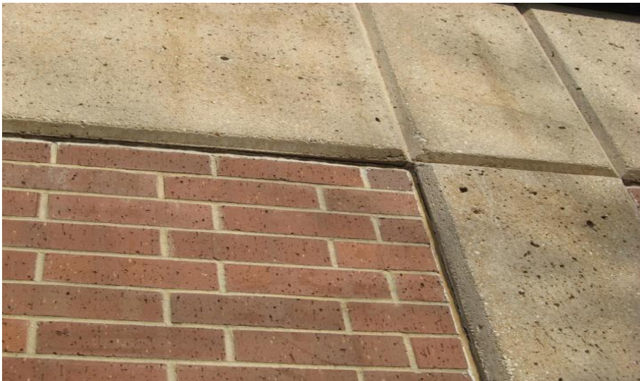
PHOTO 11 SEALANT FAILURE (MASONRY TO CONCRETE COLUMN)
