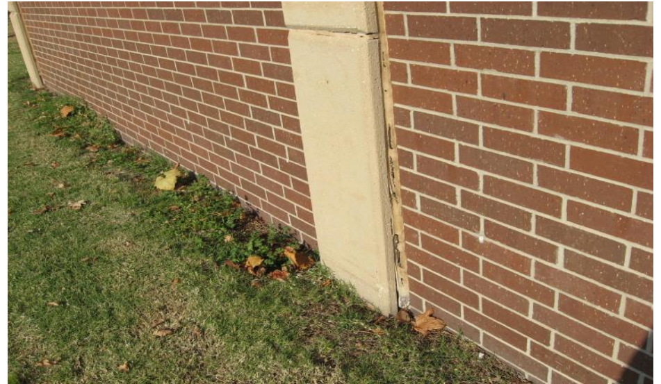
PHOTO 34 POSSIBLE PRECAST VENEER CONNECTION FAILURE
