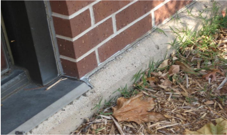
PHOTO 5 WINDOW FLASHING/MASONRY JOINT FAILURE
