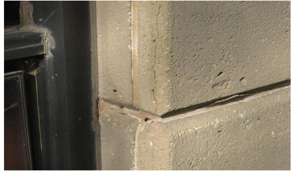
PHOTO 30 CRACKED PRECAST VENEER AT ADDITION AND SEALANT FAILURE
