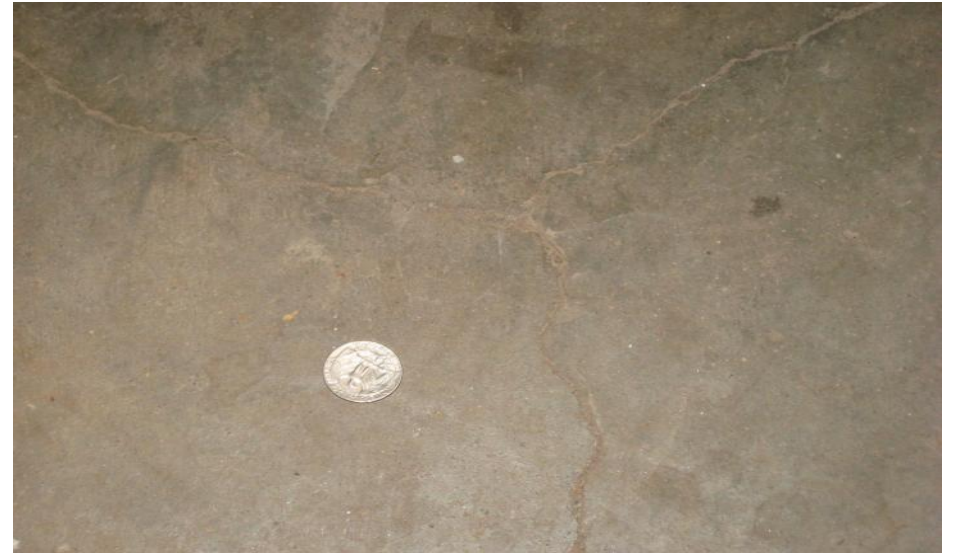
PHOTO 2 SLAB ON GRADE CRACKING AT BASEMENT
