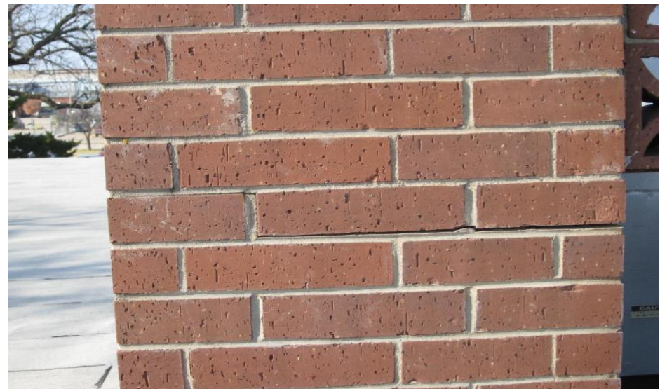
PHOTO 28 CRACKED PILASTER JOINT
