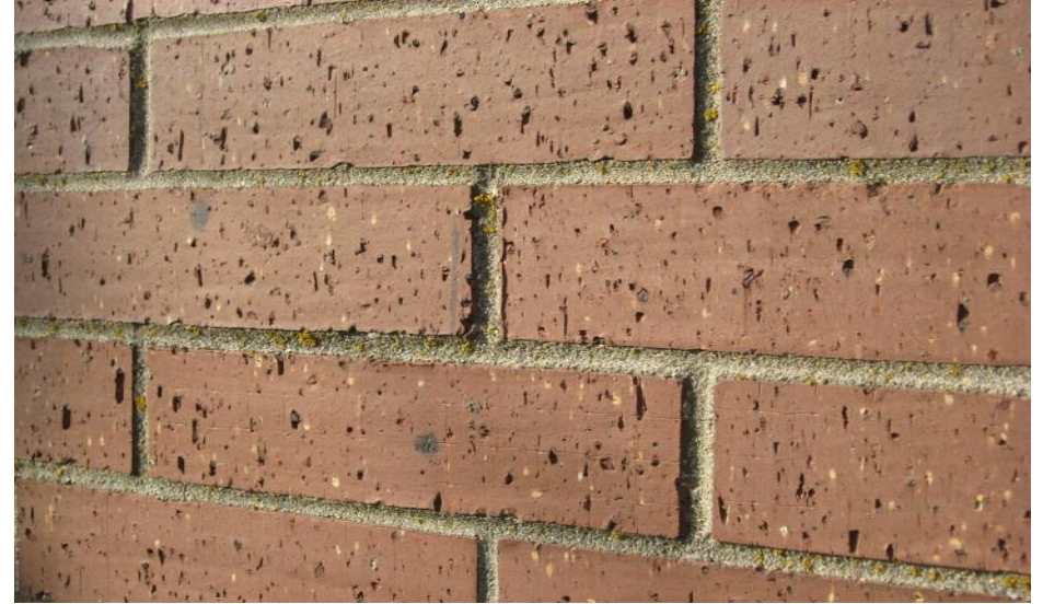
PHOTO 38 MOLD ON BRICK MORTAR SURFACE
