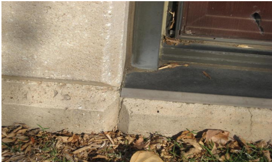
PHOTO 15 WINDOW FLASHING CRACKED CONCRETE SILL
