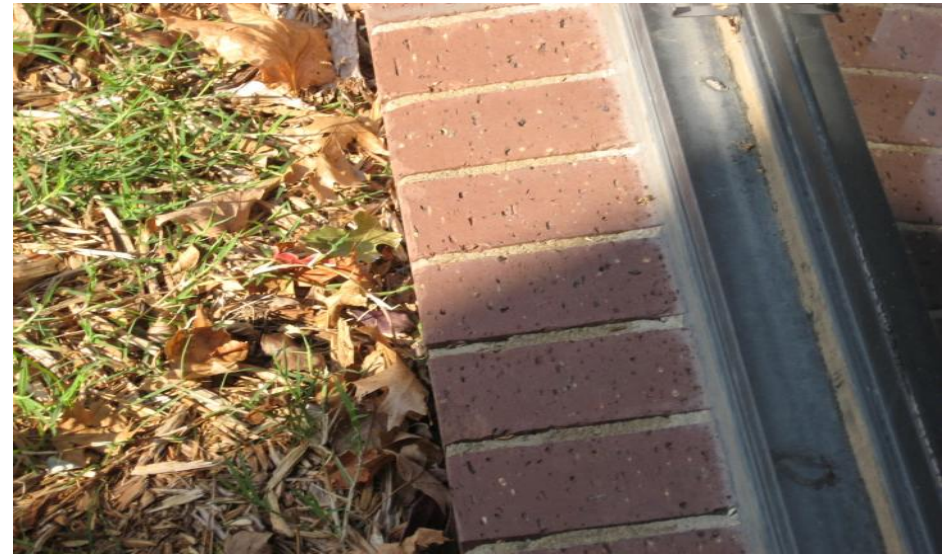
PHOTO 42 MORTAR DETERIORATION AT WINDOW SILL
