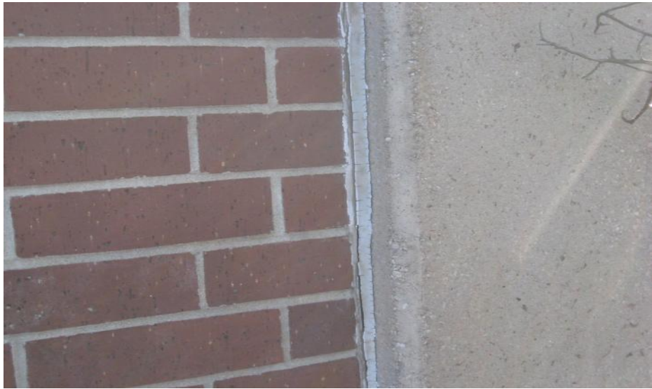
PHOTO 13 SEALANT FAILURE BRICK TO COLUMN
