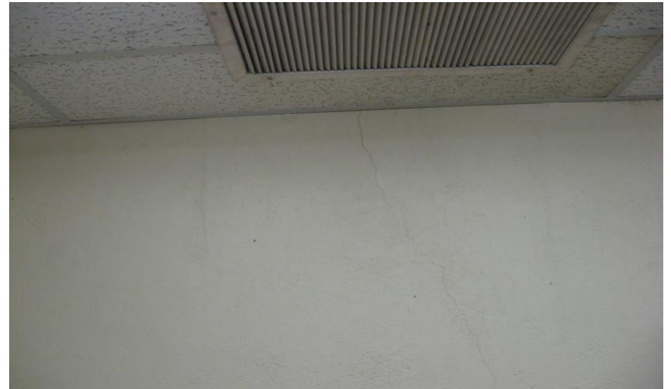
PHOTO 4 BASEMENT WALL CRACKING NEAR AN AREAWAY OPENING
