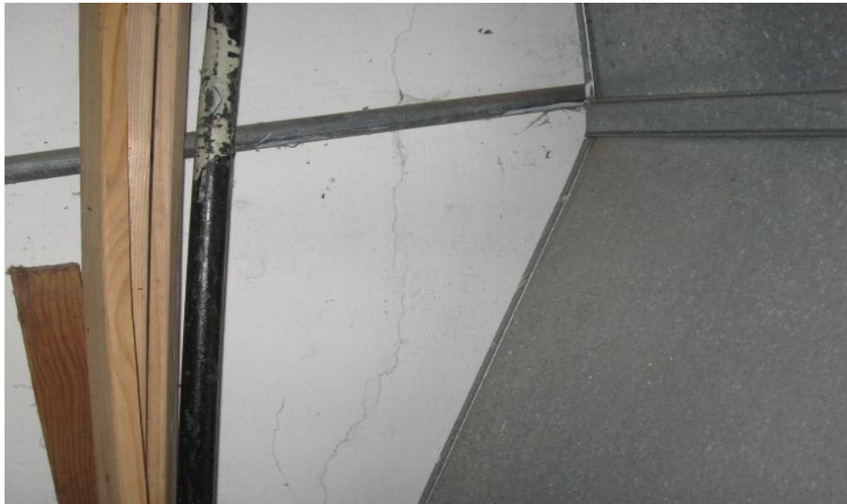
PHOTO 3 BASEMENT WALL CRACKING NEAR AN AREAWAY OPENING
