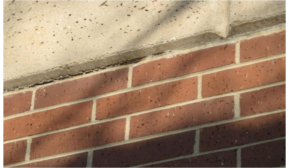
PHOTO 10 SEALANT FAILURE (MASONRY TO SPANDREL BEAM)
