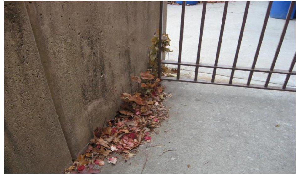
PHOTO 18 PLANT GROWTH IN OPEN SLAB JOINT
