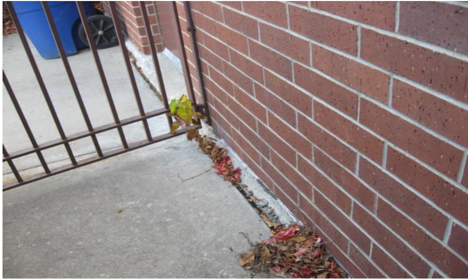
PHOTO 17 PLANT GROWTH IN OPEN SLAB JOINT
