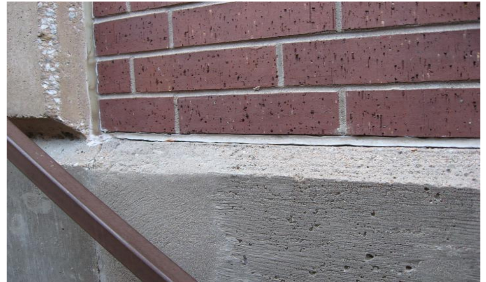
PHOTO 8 SEALANT FAILURE AT BOTTOM OF BRICK
