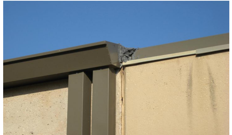
PHOTO 40 SEALANT FAILURE AT FLASHING TRANSITION
