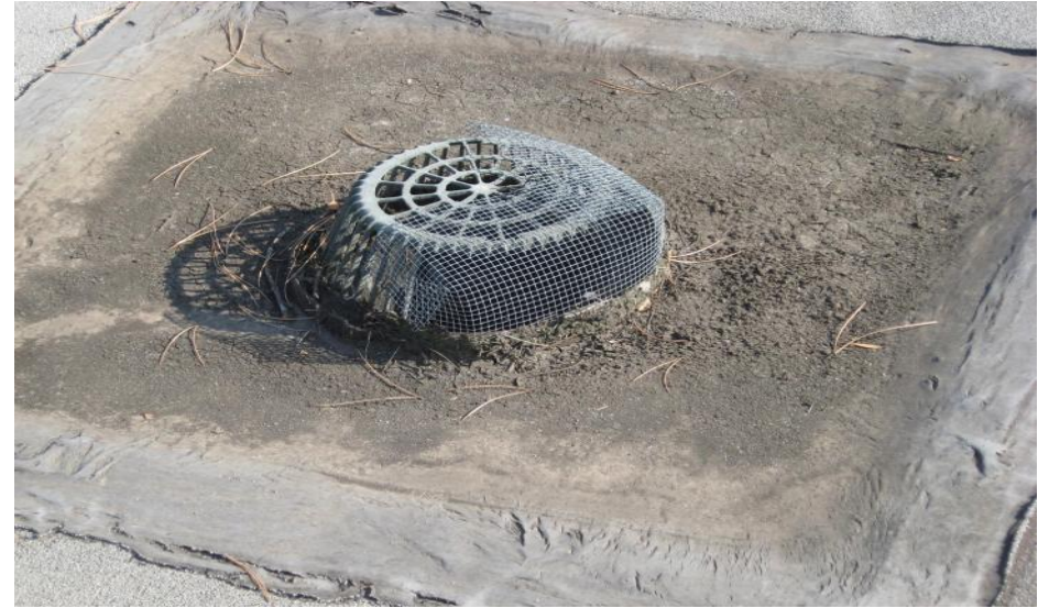
PHOTO 46 PARTIALLY BLOCKED AND BROKEN ROOF DRAIN
