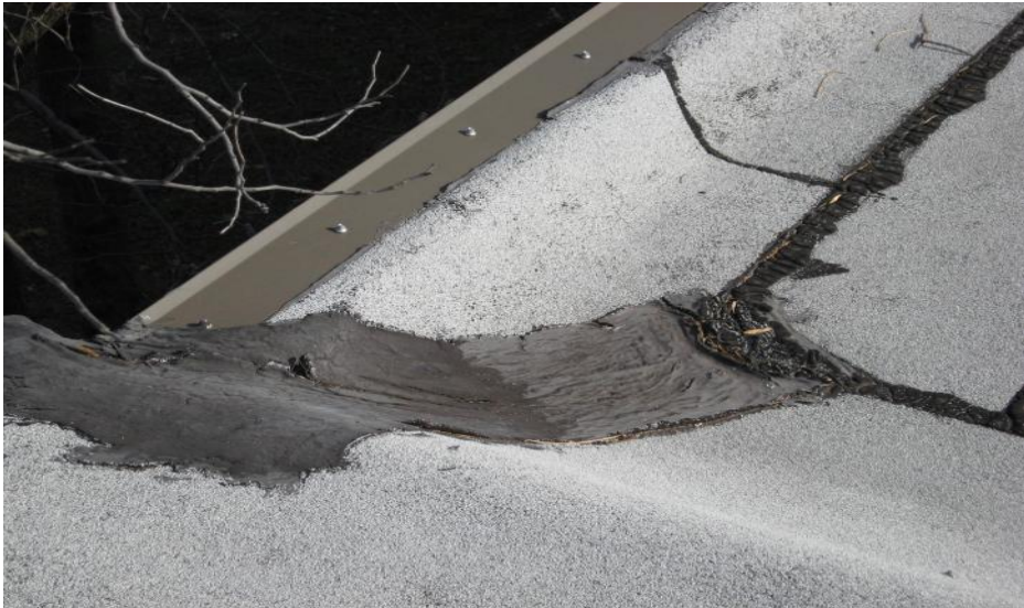
PHOTO 47 POTENTIAL ROOF LEAK AT SEALANT
