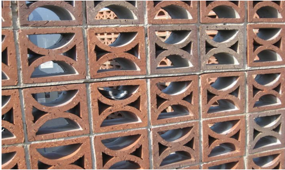
PHOTO 29 CRACKED MORTAR JOINT
