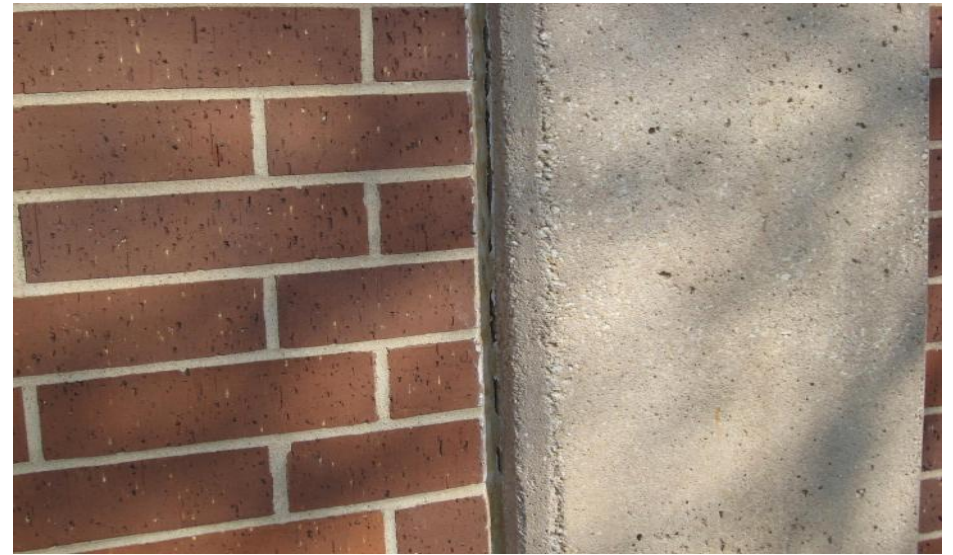
PHOTO 14 SEALANT FAILURE MASONRY TO CONCRETE COLUMN
