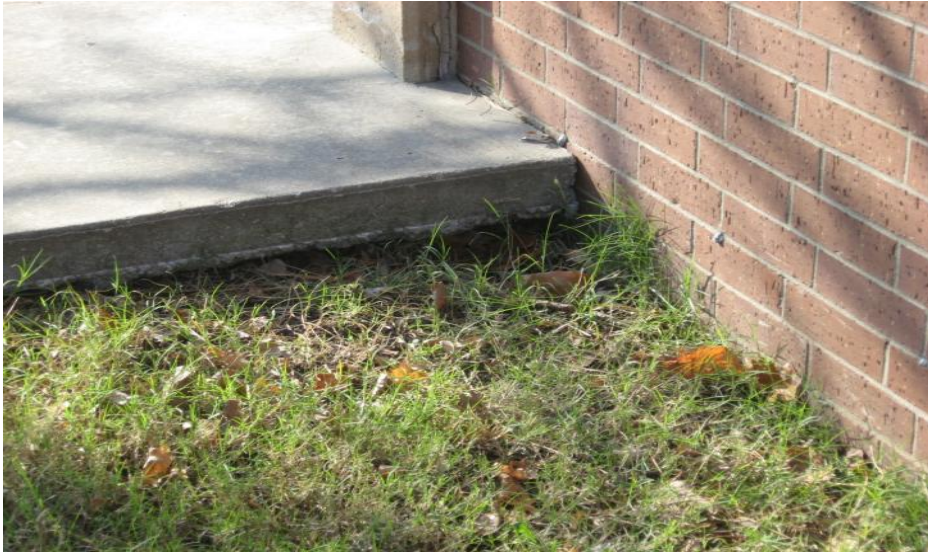
PHOTO 45 SETTLEMENT OF SOILS ADJACENT TO BUILDING AND BELOW SIDEWALK
