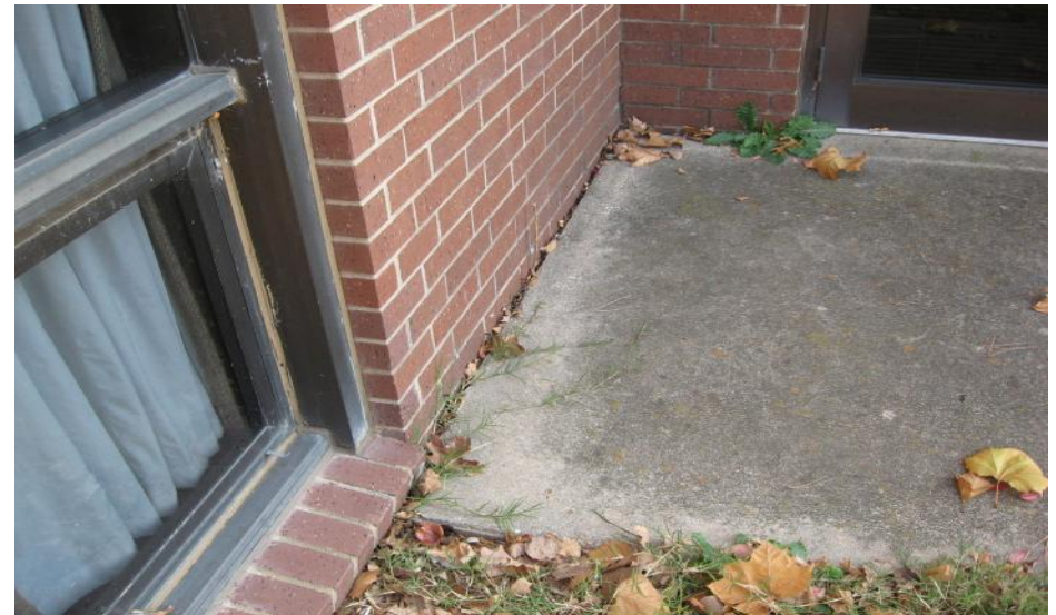
PHOTO 44 OPEN JOINT AT SIDEWALK SLAB
