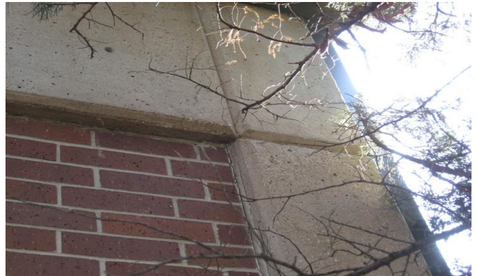
PHOTO 12 SEALANT FAILURE BRICK TO COLUMN AND BRICK TO SPANDREL
