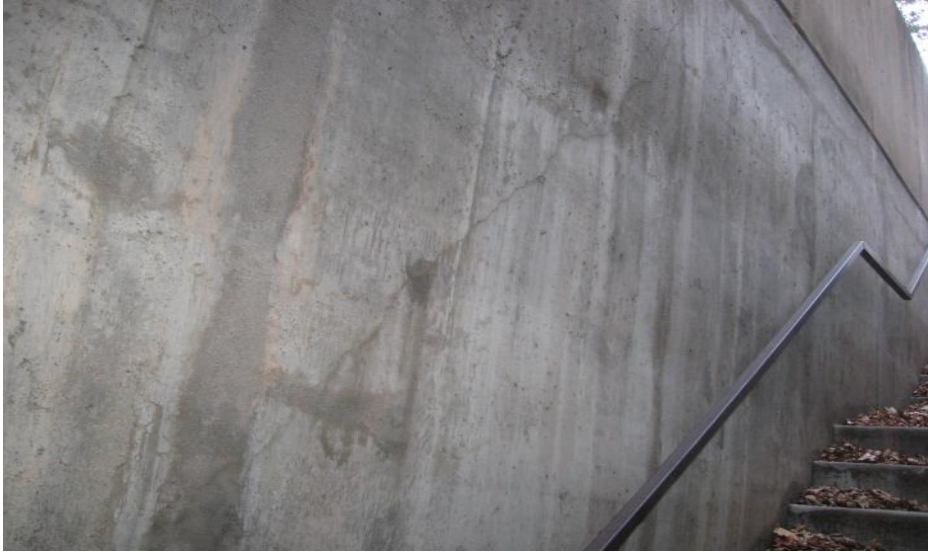
PHOTO 21 CRACKED WALL AT EXTERIOR STAIR
