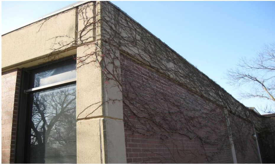
PHOTO 41 VINES ON SIDE OF BUILDING SOURCE OF MASONRY DETERIORATION
