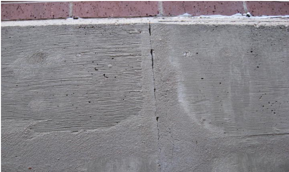
PHOTO 7 CRACKED AND OPENED CONSTRUCTION JOINT
