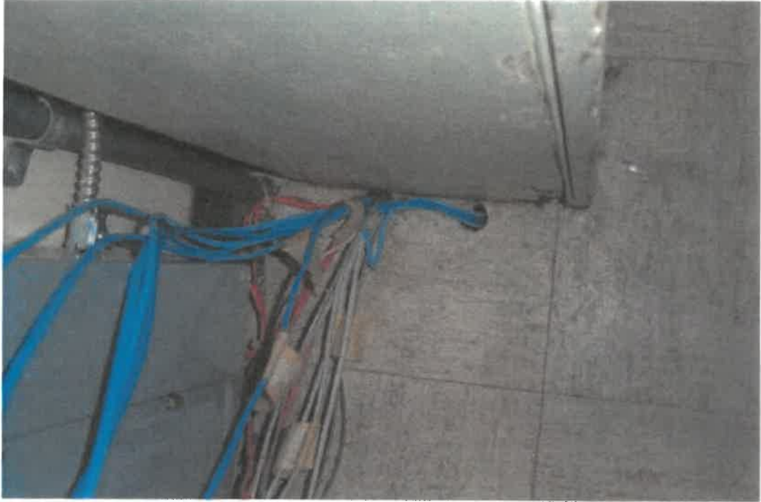
7.1.1. Non-Firestopped Openings – View 2056
