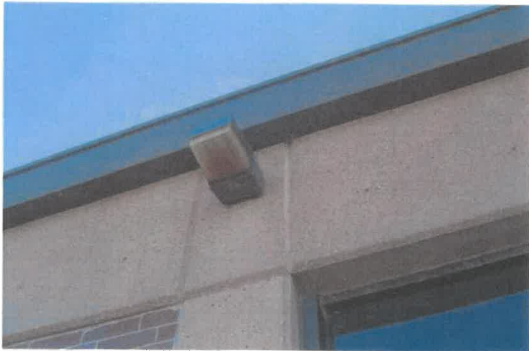
6.3.1. Exterior Light Fixture - View 1940-1
