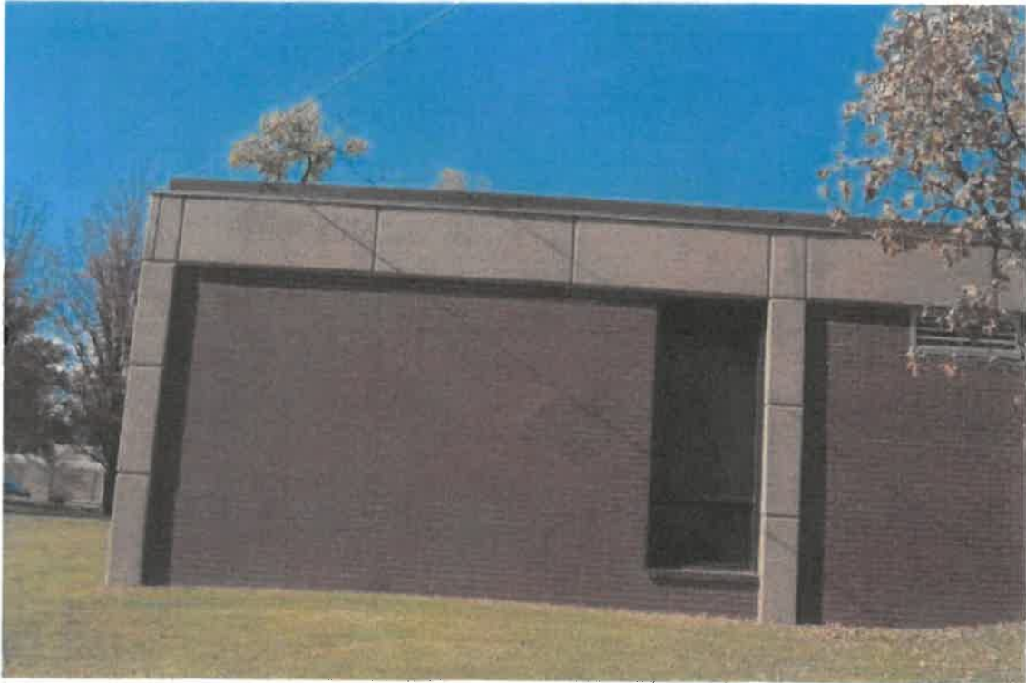
5.1.3. Service Lines Above Roof - View 1961
