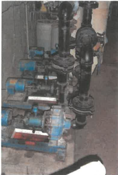
4.3.5. Hot & Chilled Water Pumps – View 1996-1
