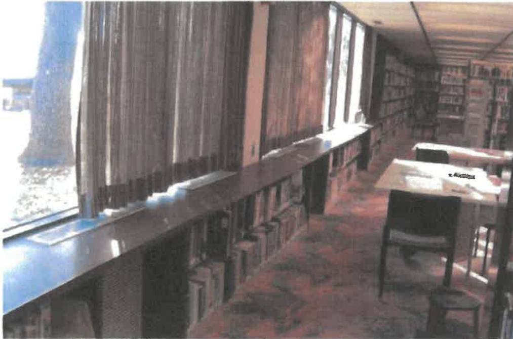
4.2.3.2. Fin-Tube Window Heat – View 2060
