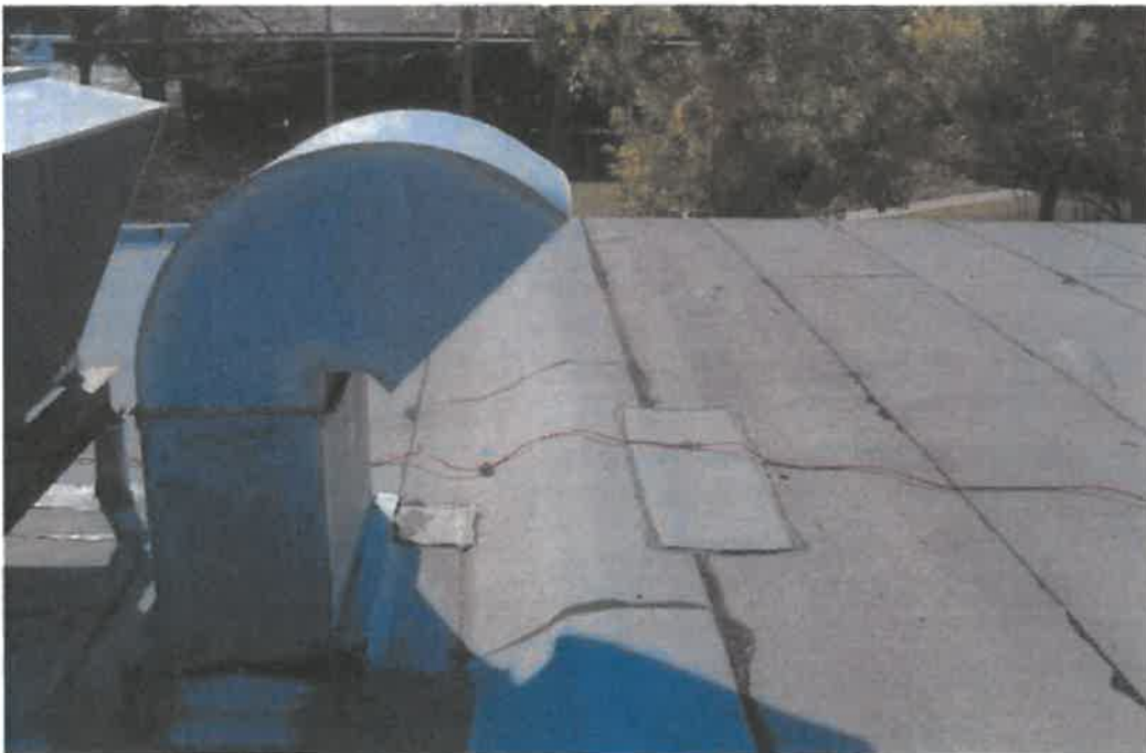
4.1.1.3. - Fresh Air Intake Hood - View 1897
